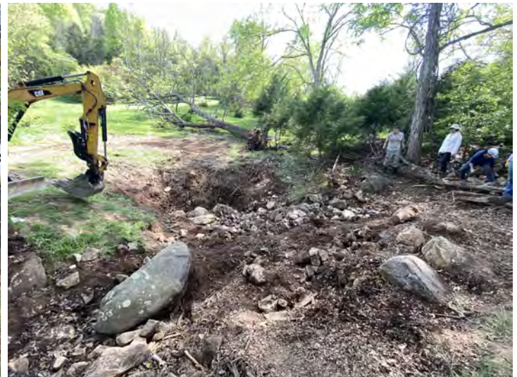
Heavy equipment was used for the Bland County Sinkhole Cleanup. Photo by Meredith Weberg
