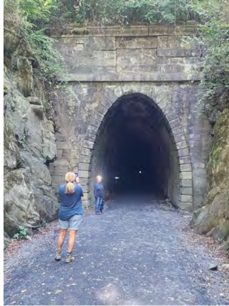
The Western (Blue Ridge) entrance to the tunnel with Cyndi Hutchison and Mary Sue Socky. (note 1850's masonry) Photo by Barry Ferguson
